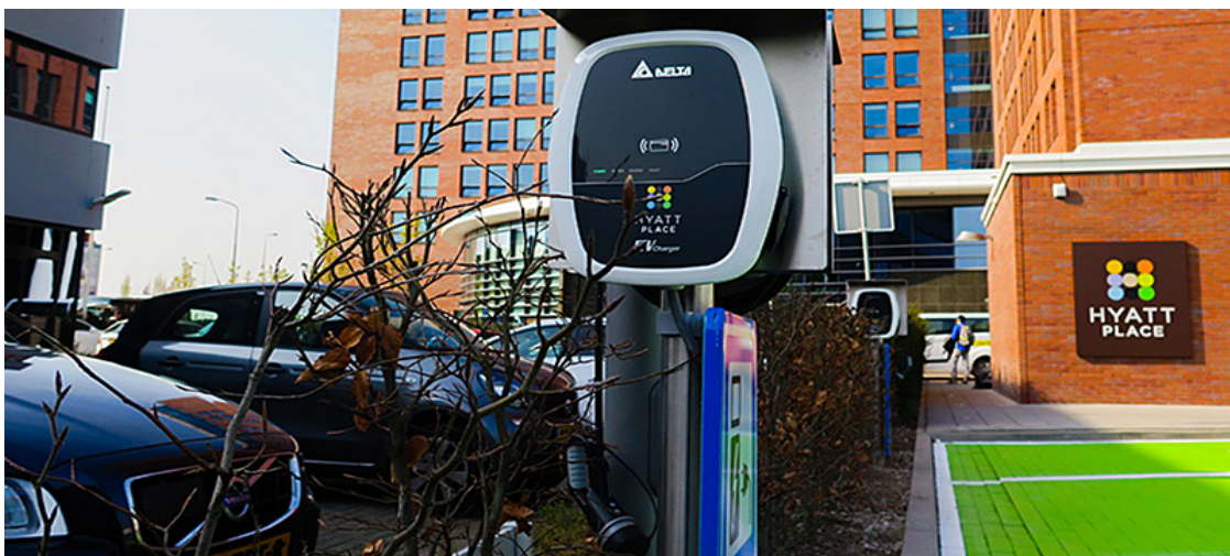
Figure 14 EV Chargers for Hyatt Airport Hotel in Amsterdam, the Netherlands
