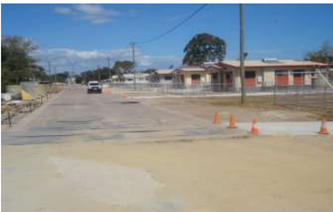
New paving takes you to the Pormpuraaw State School. Raaku Street on the Northside subdivision benefits from the work. (Photographs: Ian Anders, DATSIP).
