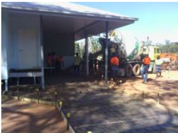
Members of the civil work team delivering new housing in Napranum. (Photographs: (left) courtesy of the Napranum Aboriginal Shire Council and (right) supplied by Katrina Beattie, DATSIP).
