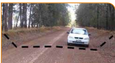
Figure 14.16: Subsurface road from which runoff cannot escape
