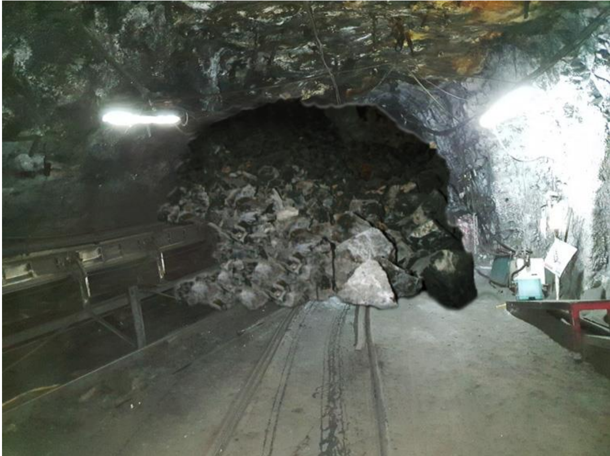
Figure 6 Roof fall at the bottom of the dolly car drift
