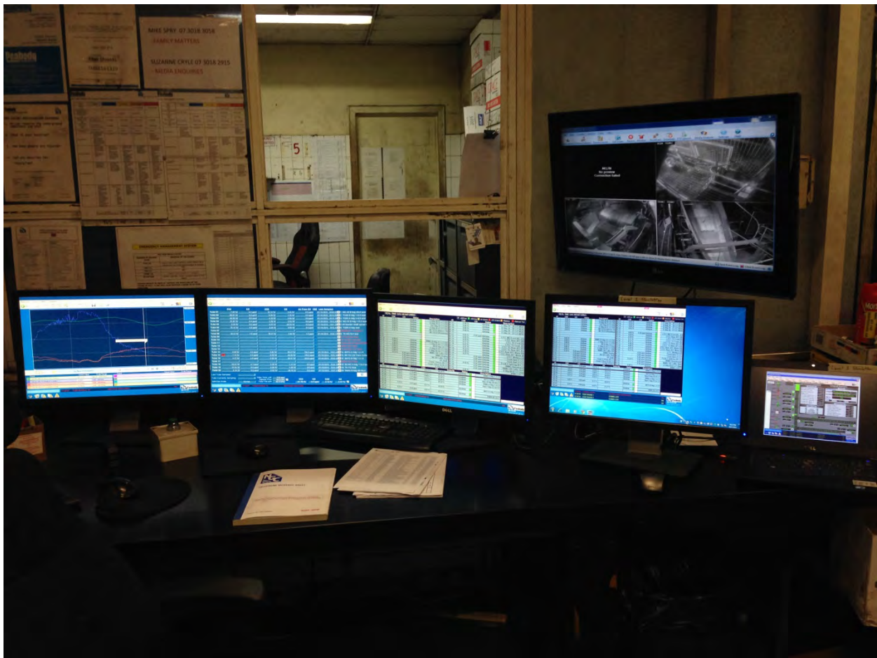
Figure 6: Computer layout in the control room
