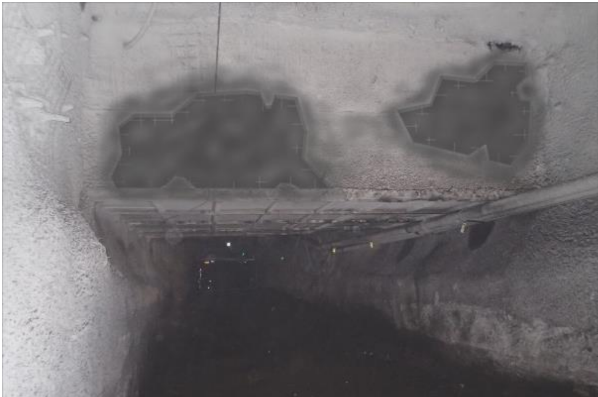
Figure 6 damaged 9 c/t overcast
