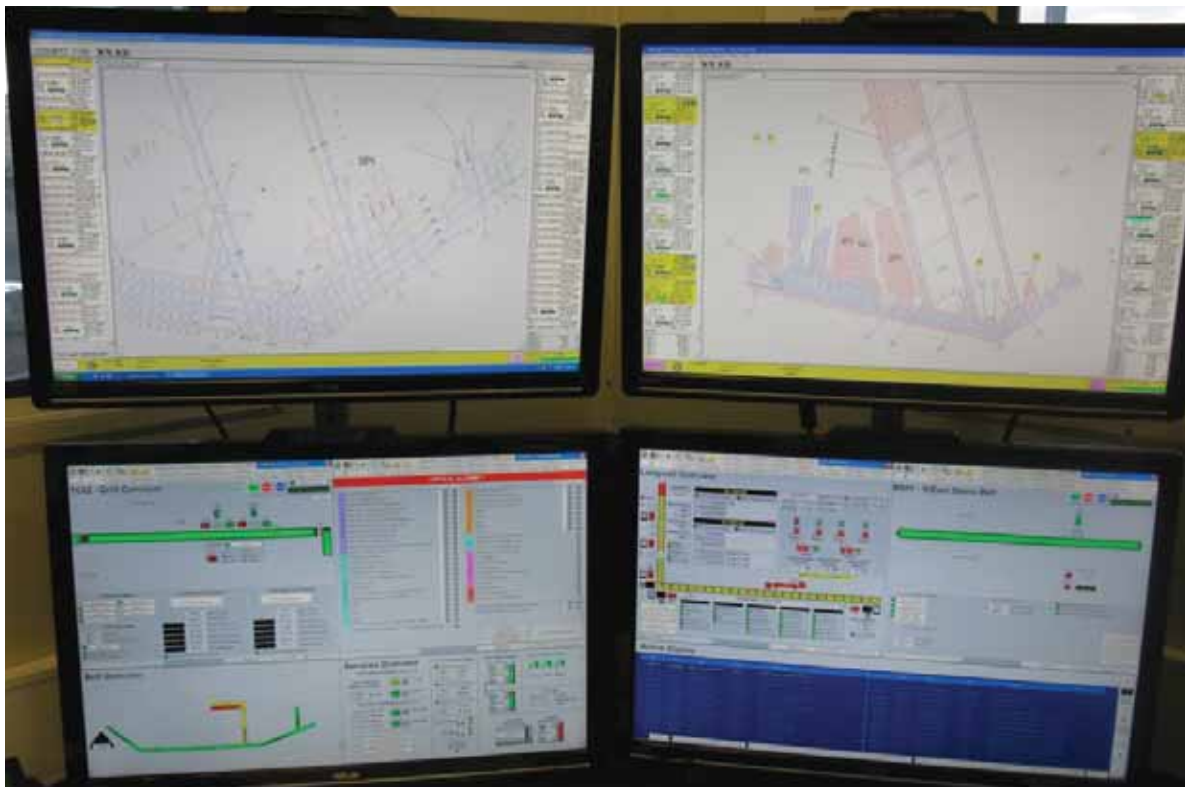
Communications Room, Carborough Downs Coal
