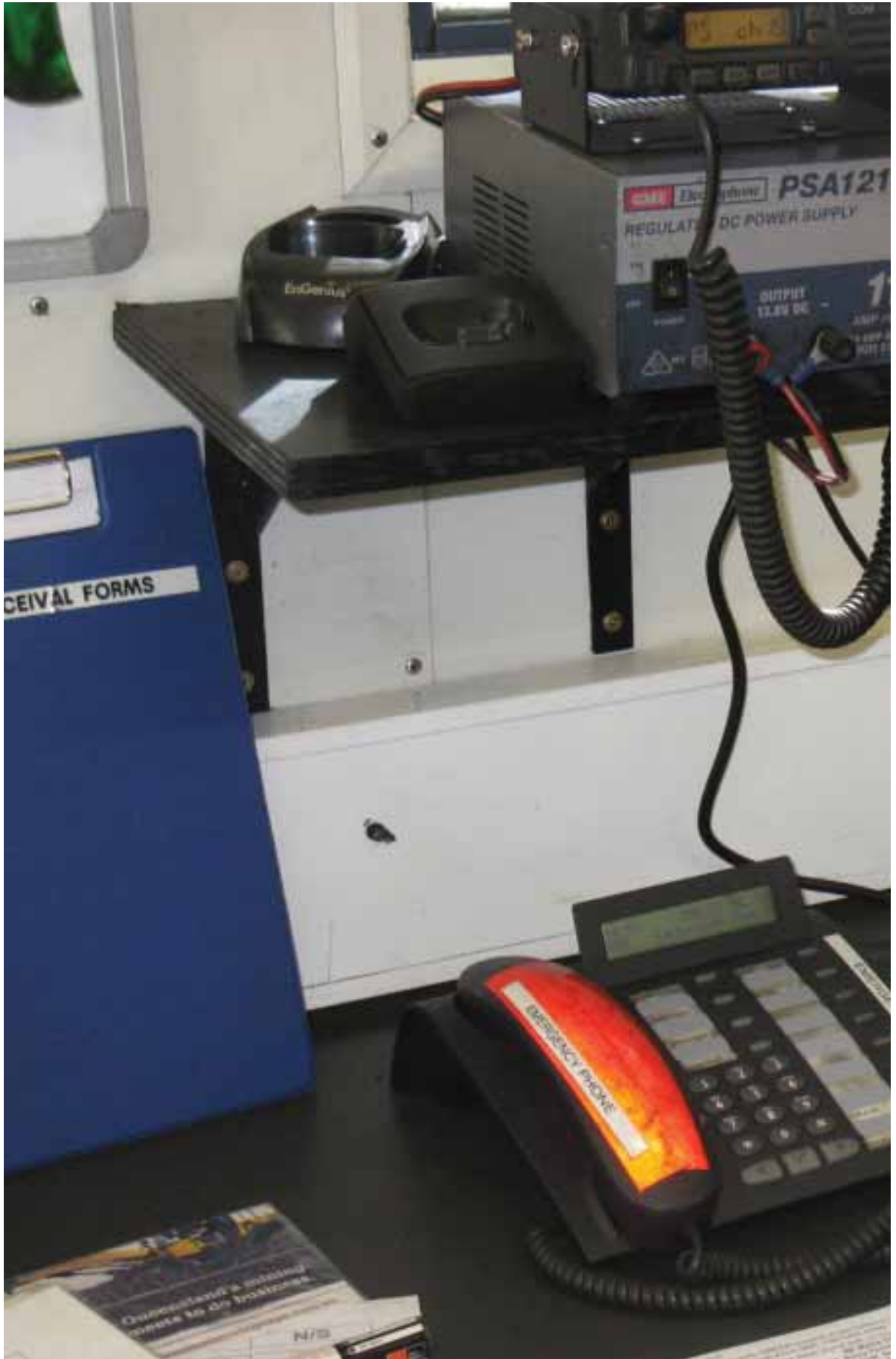
Communications Room, Carborough Downs Coal
