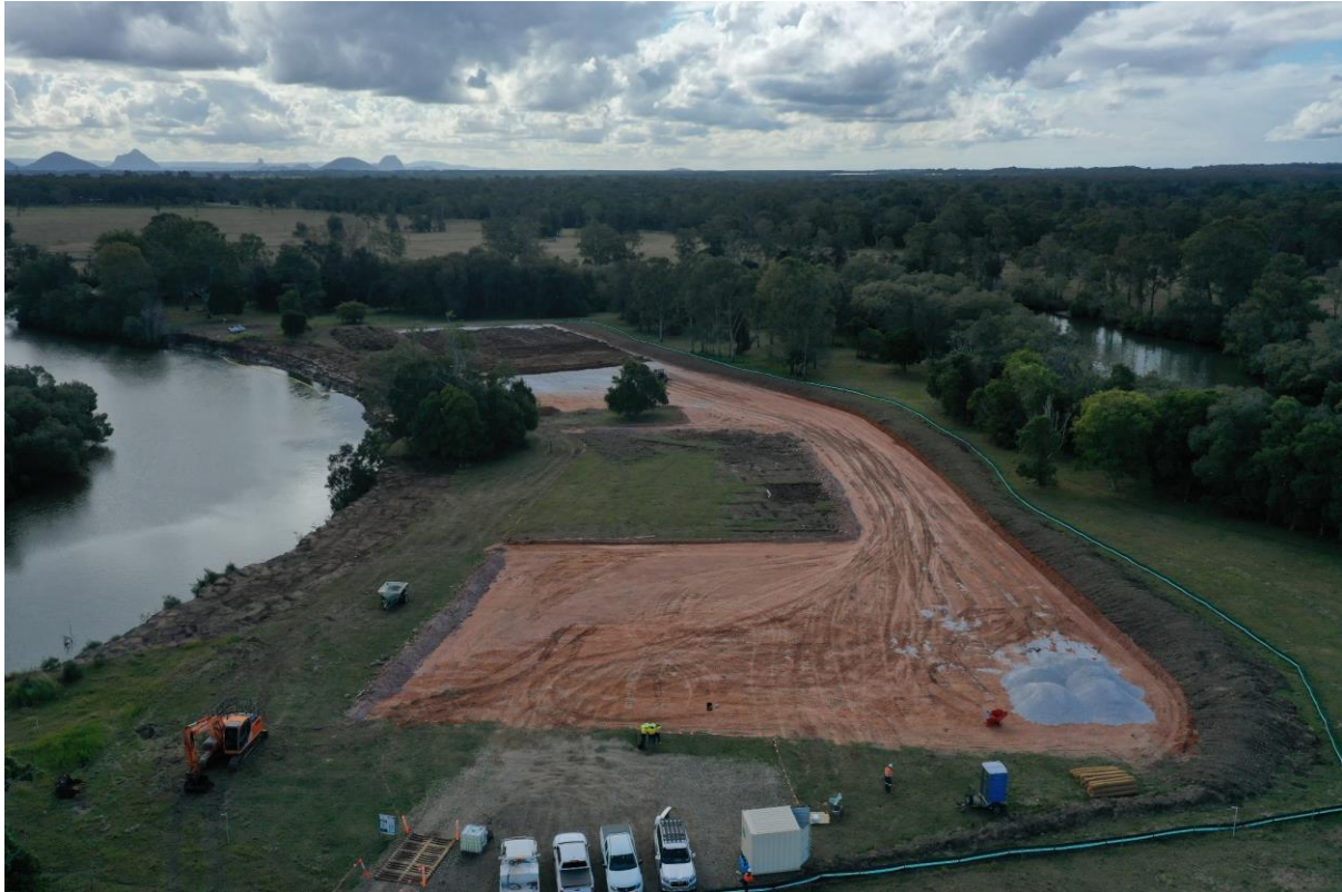
Figure 6: ASS treatment pad in South East Queensland
