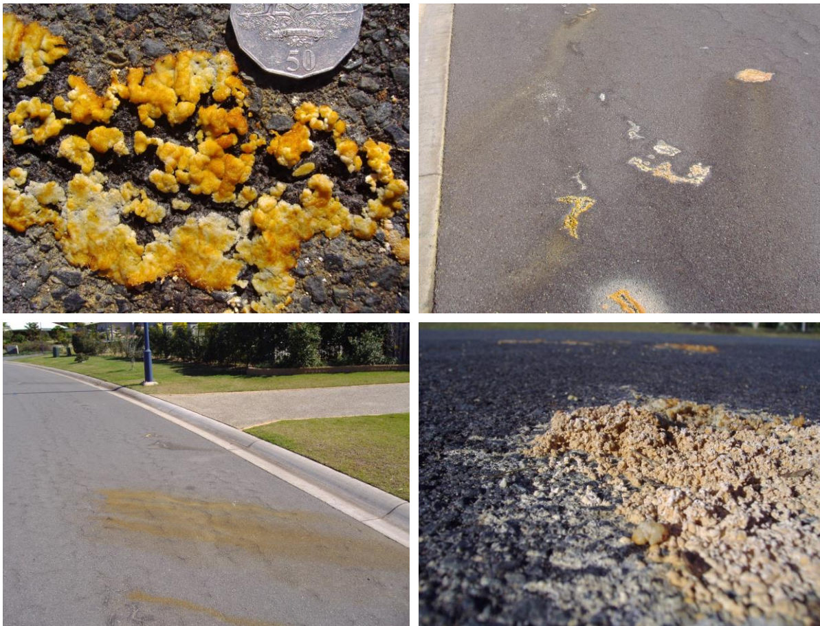
Figure 16: Acidic salts and minerals on asphalt surfaces
