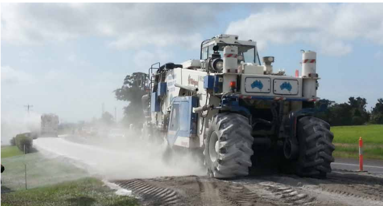
Foamed bitumen is more durable and cost effective compared to asphalt concrete.
