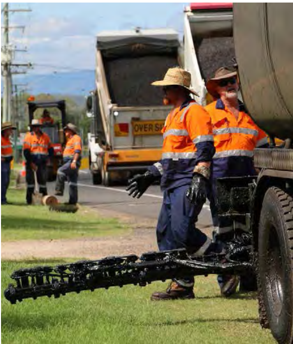
A new plan for old tyres—the crumb rubber modified road seal could potentially replace conventional bitumen seals.
