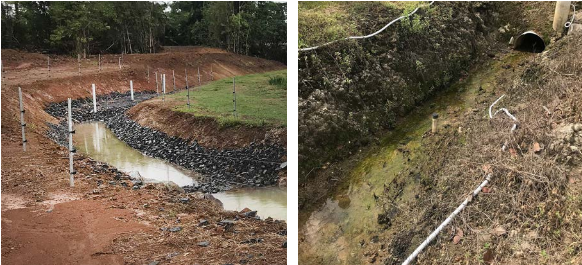
Figure 1.15 Bioreactor beds installed downslope of cane farms in the Wet Tropics region. Photo on left shows in-line bioreactor bed above the floor of the drain. Photo on right shows in-line bioreactor bed below the floor of the drain.
