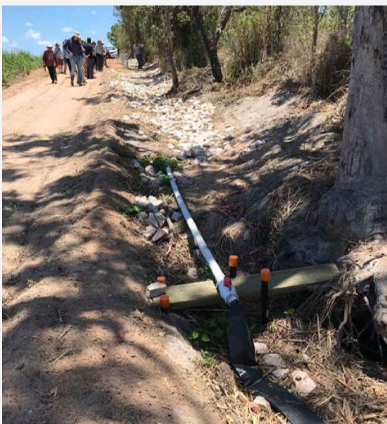
Figure 3 Bioreactor outlet showing single outlet pipe with valve to regulate flow, if required.
