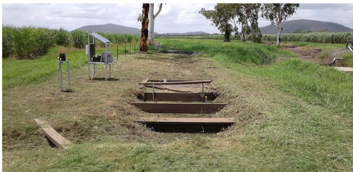
Figure 3.7 Sediment basin shown in the foreground with baffles to slow water velocity and enable sediment to settle before water flows into the bioreactor (beyond timber sleepers).
