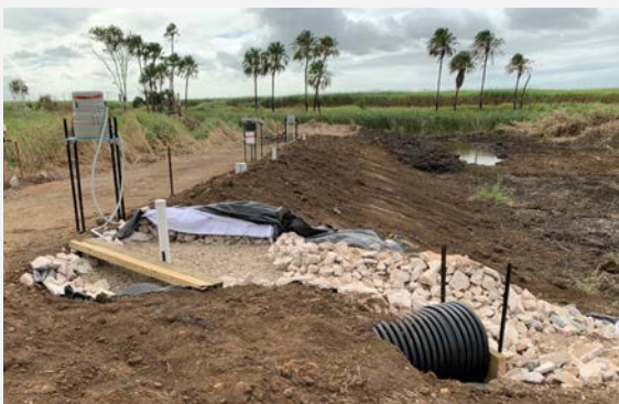
Figure 3 Completed bioreactor showing inlet structure with pipe from upslope cane block directing water into the inlet pit filled with washed river gravel (left). Excess flow bypasses the structure to a low-lying area on the right.
