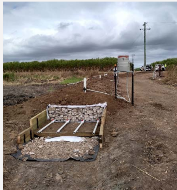
Figure 4 Bioreactor outlet showing four outlet pipes.
