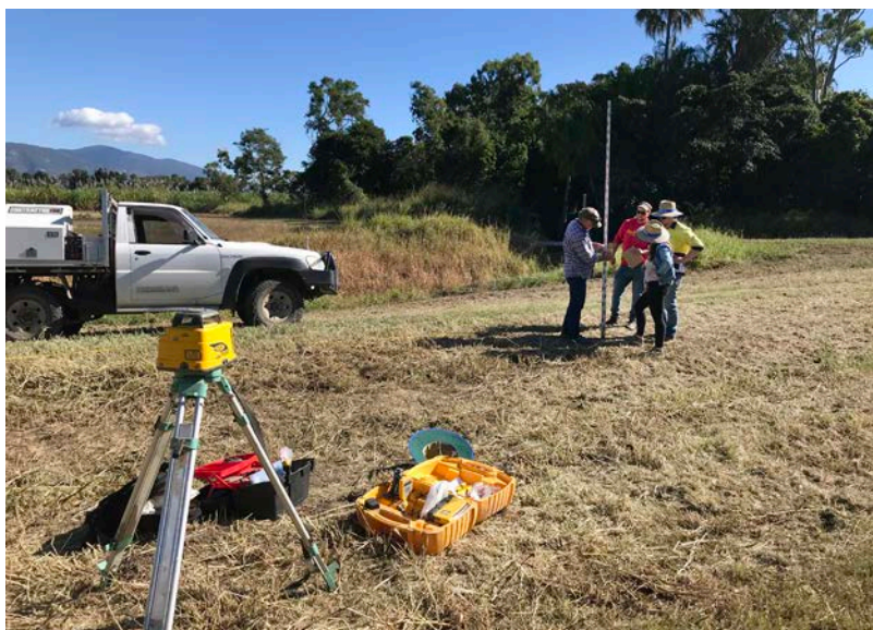
Figure 3.1 Taking levels during the site investigation to determine if slope is sufficient.
