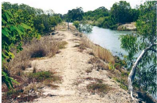
Photograph 27: AASS that has formed on the bank of a prawn farm intake channel excavated across mangrove flats at McEwens Beach
