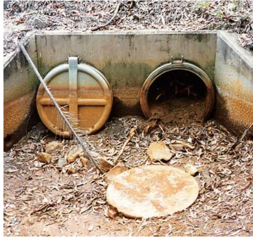
Photograph 5: Concrete infrastructure displaying pitting due to attack by acidified drainage water
