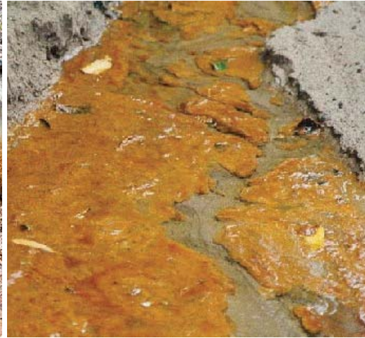
Photograph 6: Iron oxides choking a drain
