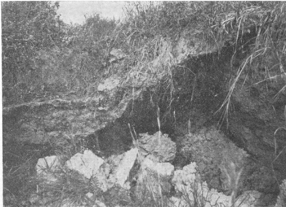
Fig. 8. Typical failure of a scour check. In this case it has been undermined and by-passed.
