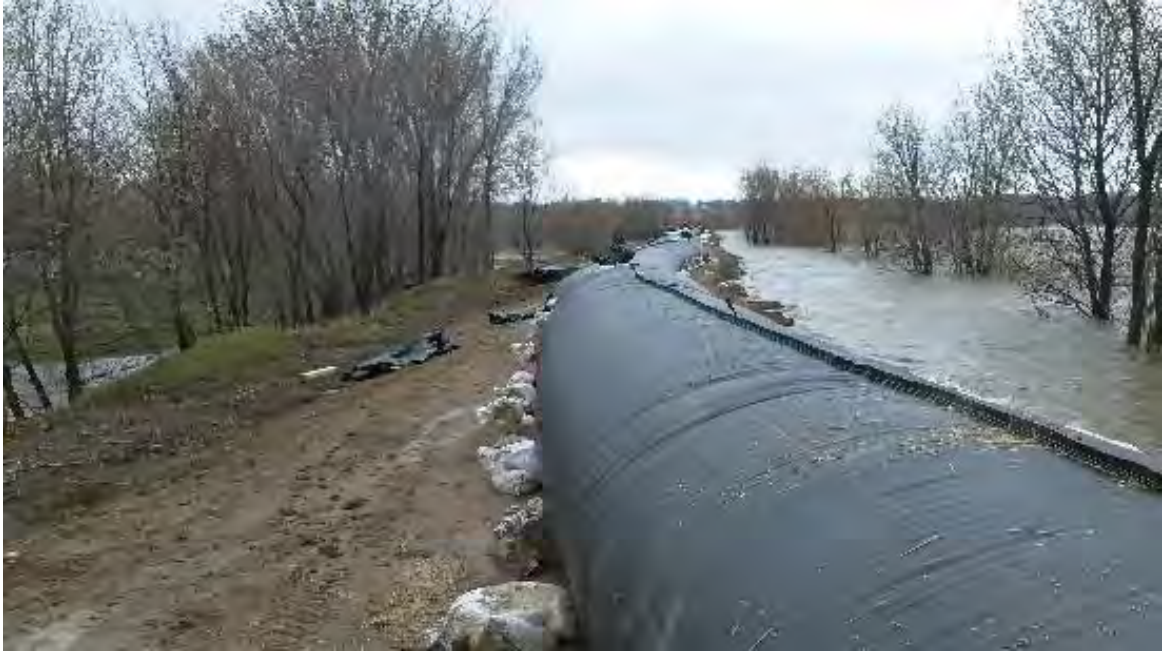
Figure 8-36 Water-filled tube flood barrier [ www.readreidread.wordpress.com/ ]
