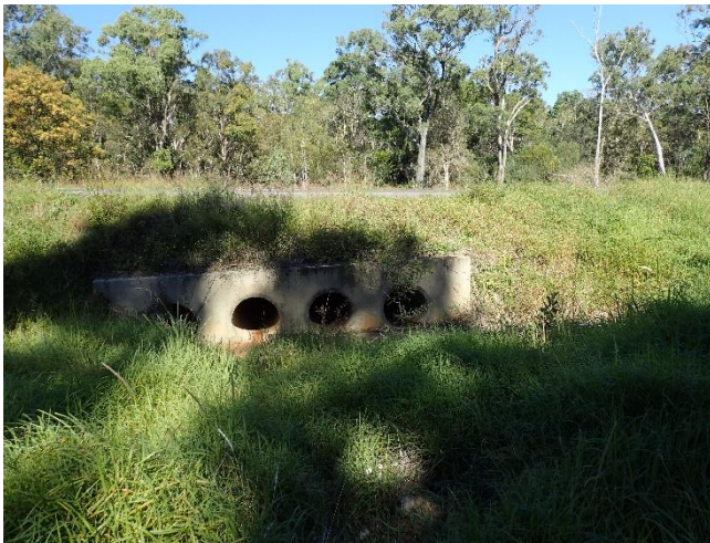
Figure 10 Four pipe road culvert in wetland inlet/outlet channel (C. Johns, 2017). While there are four pipes here, these are contained in the one structure and should be counted as a single point inflow.
