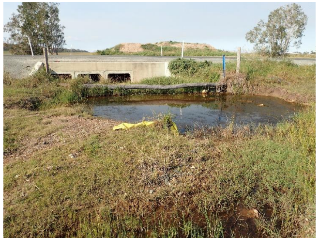
Figure 11 Roadway box culvert into wetland (C. Johns, 2017). While there are three pipes here, these are contained in the one structure and should be counted as a single point inflow.
