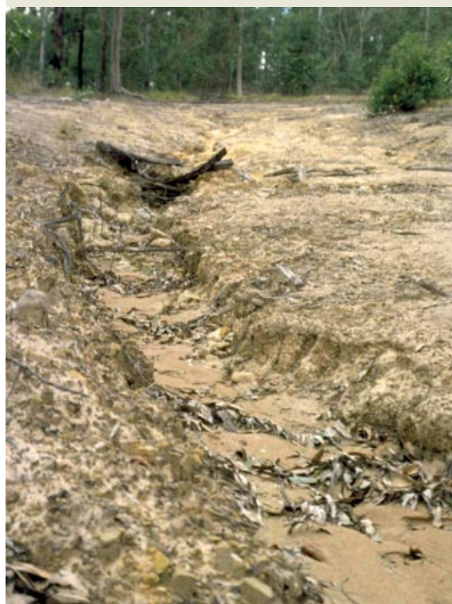
Figure 2.10 A badly eroded access track. Erosion can be avoided by post-harvest draining all snig and haulage tracks.
