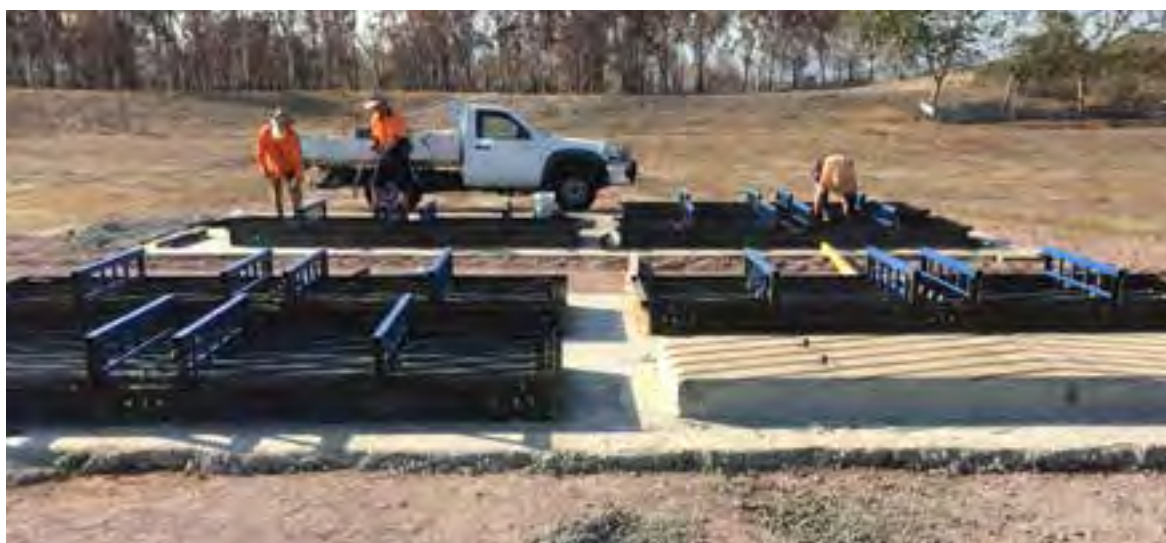
Precast structures manufactured for the reconstruction of Wallace Landing boat ramp and the BP Home Hill access reconstruction by the department saved money and time.
