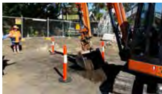
Creating 31 parking spaces at the Salisbury Park 'n' Ride, whilst looking after the environment.
