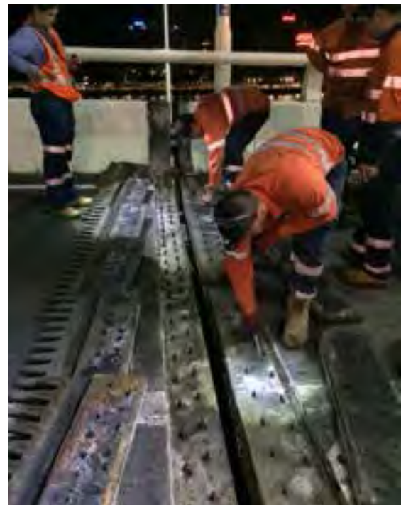
New work practices including the custom design tooth to clean bridge joints.
