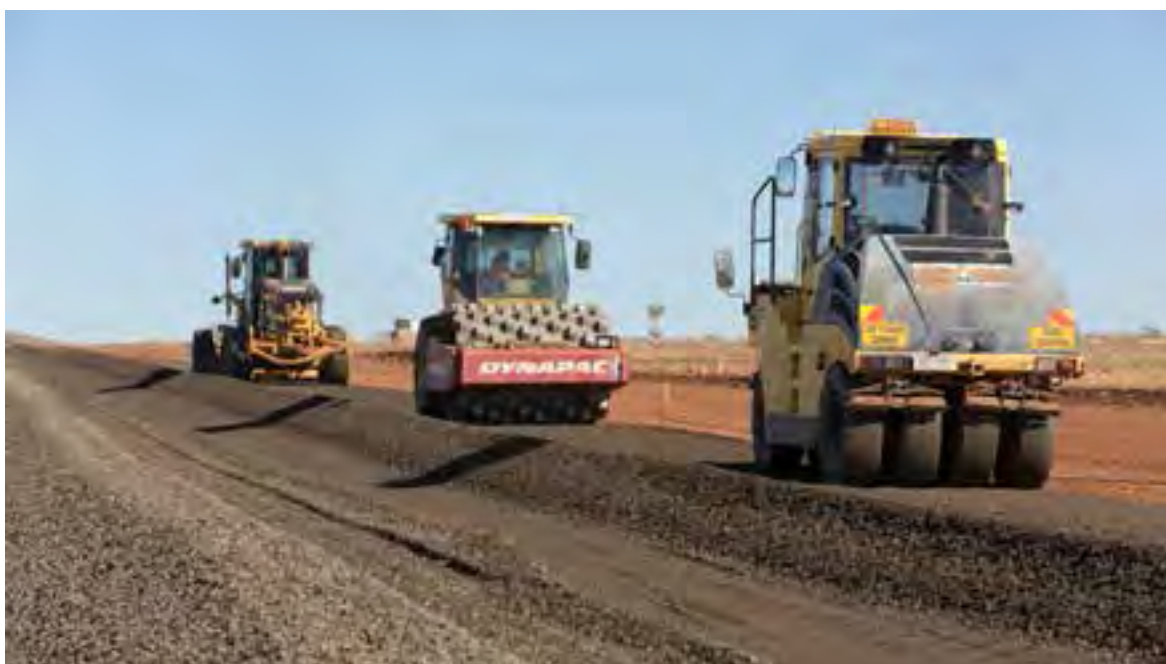
Plant in operation on the Cloncurry-Dajarra Road (Cloncurry-Duchess) as part of the Western Roads Upgrade Program
