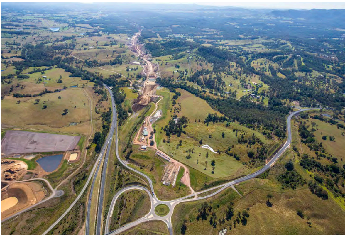
Progress on Cooroy to Curra Section C – looking north from Traveston interchange (June 2016)
