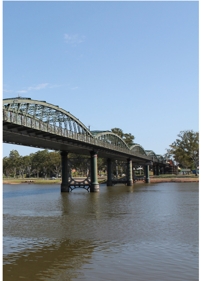
The steel girder bridge has eight spans and is 416 metres in length between abutments. It was officially opened by the Queensland Governor Baron Lamington on 24 August 1900.
