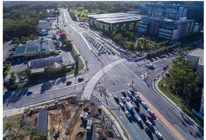
Aerial view of stage two construction at Olsen Avenue and Wintergreen/Parklands Drive intersection.
