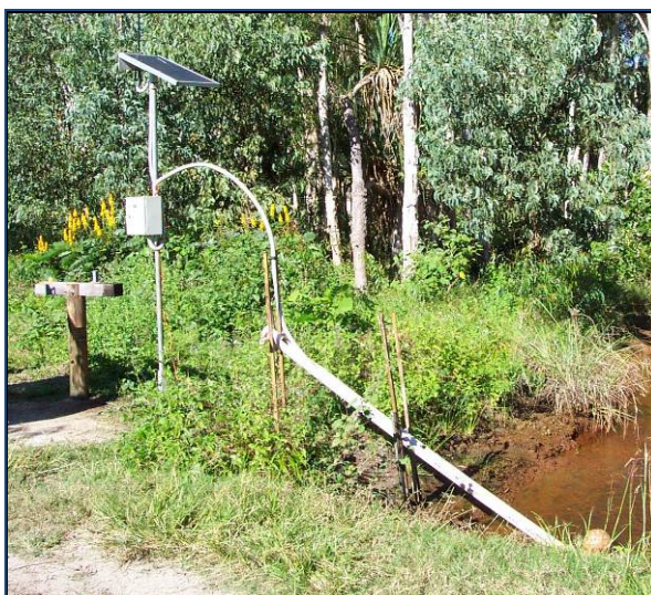
Figure 3 – An automated water quality monitoring system with pH, temperature and conductivity meters, a data transmitter and independent power source (solar panel and backup battery). Systems like this require cleaning and calibration around once per week and their output can be monitored remotely.
